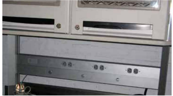
Double Raceway attached to a mobile Starsys system.
